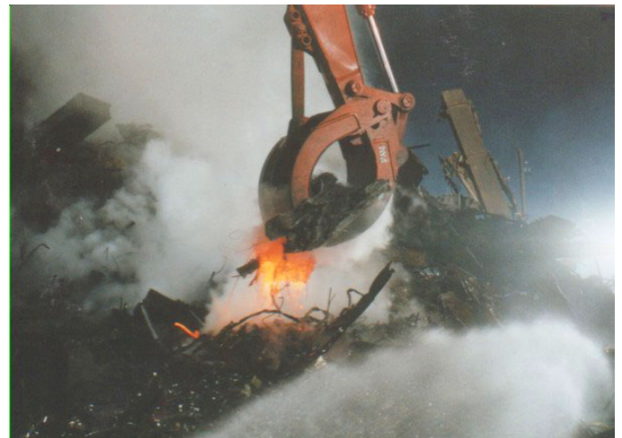
Figure 7: An excavator picks up metal rubble from deep within the pile, and some of it is dripping a yellow-white hot liquid metal at or above 1,200°C/2,200°F. This is approximately double the temperature that can be reasonably expected from an oxygen-starved fire.
